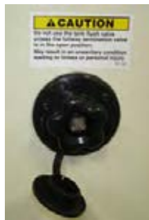
Tank Flush Inlet
